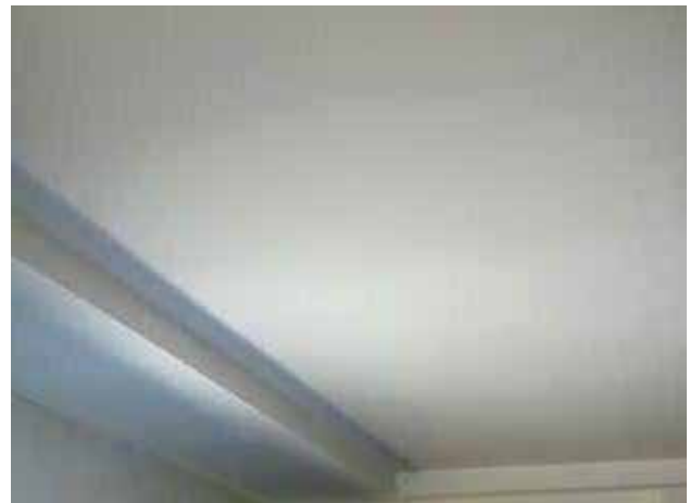
Bulk Head False Ceiling
